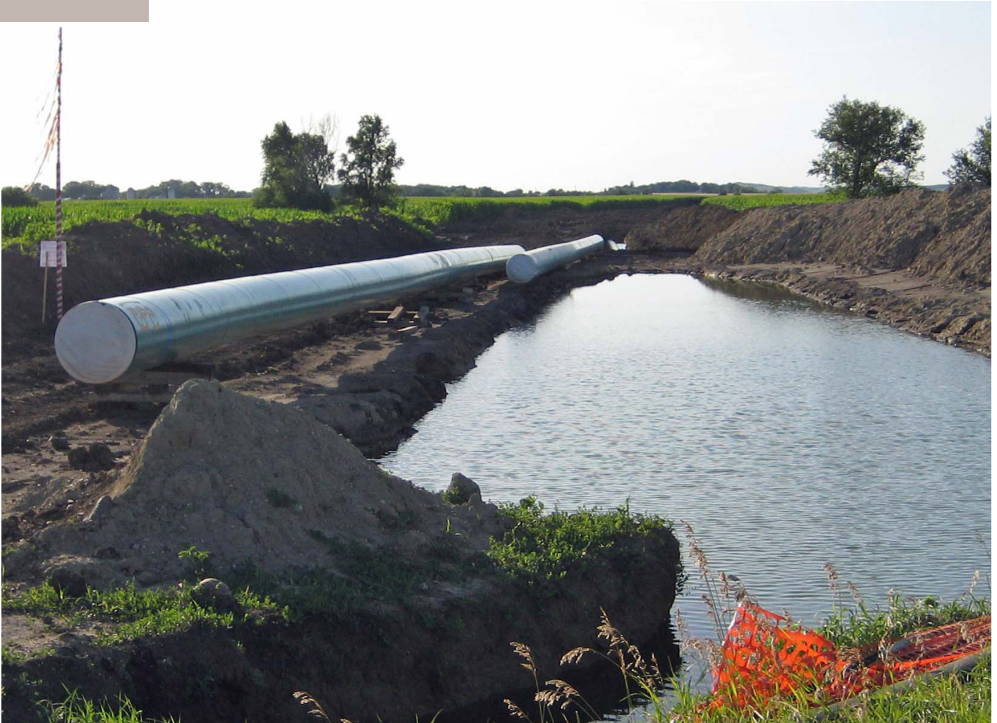
Construction of pipeline near Yankton, South Dakota in 2009. Photo courtesy of Tar and Pipelines at Wordpress
